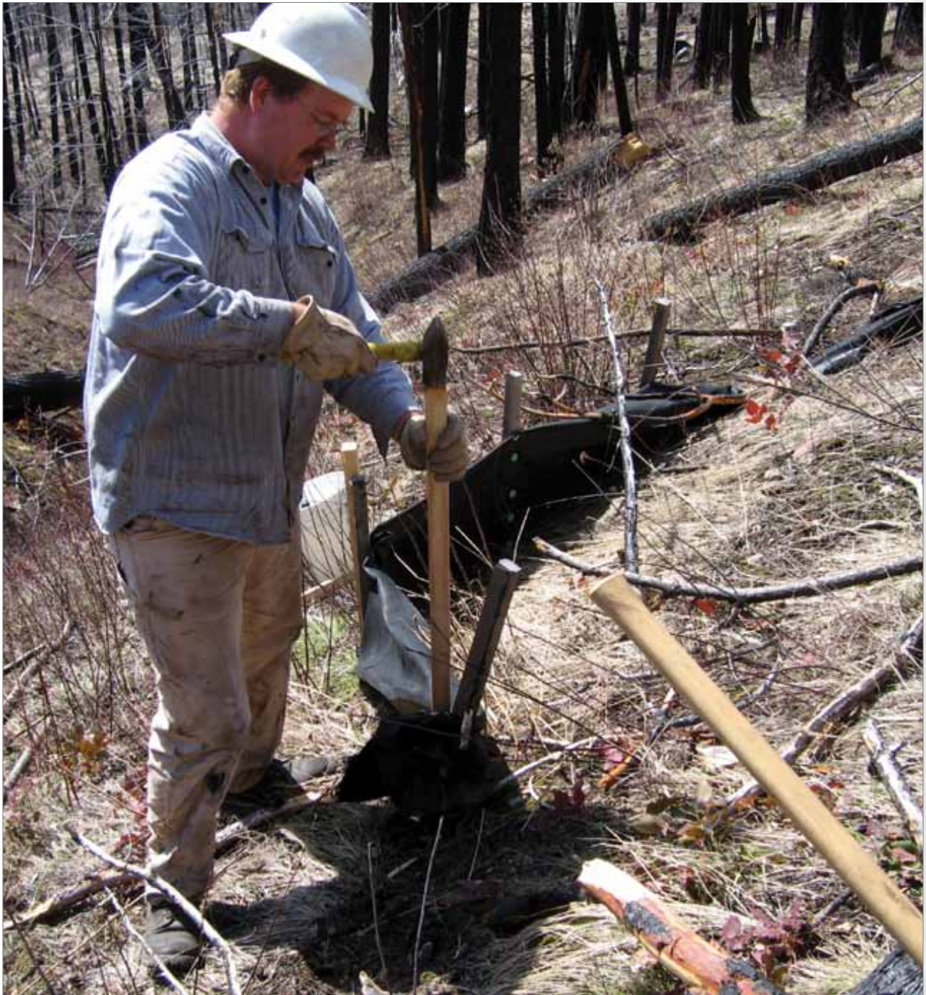
Bob Brown, hydrologist with the U.S. Department of Agriculture Forest Service, repairs a silt fence after the 2003 Myrtle Creek Fire on the Idaho Panhandle National Forest. The silt fences in this area were used to measure the effectiveness of straw mulch, hydromulch, and natural needle cast on reducing erosion after the fire.
